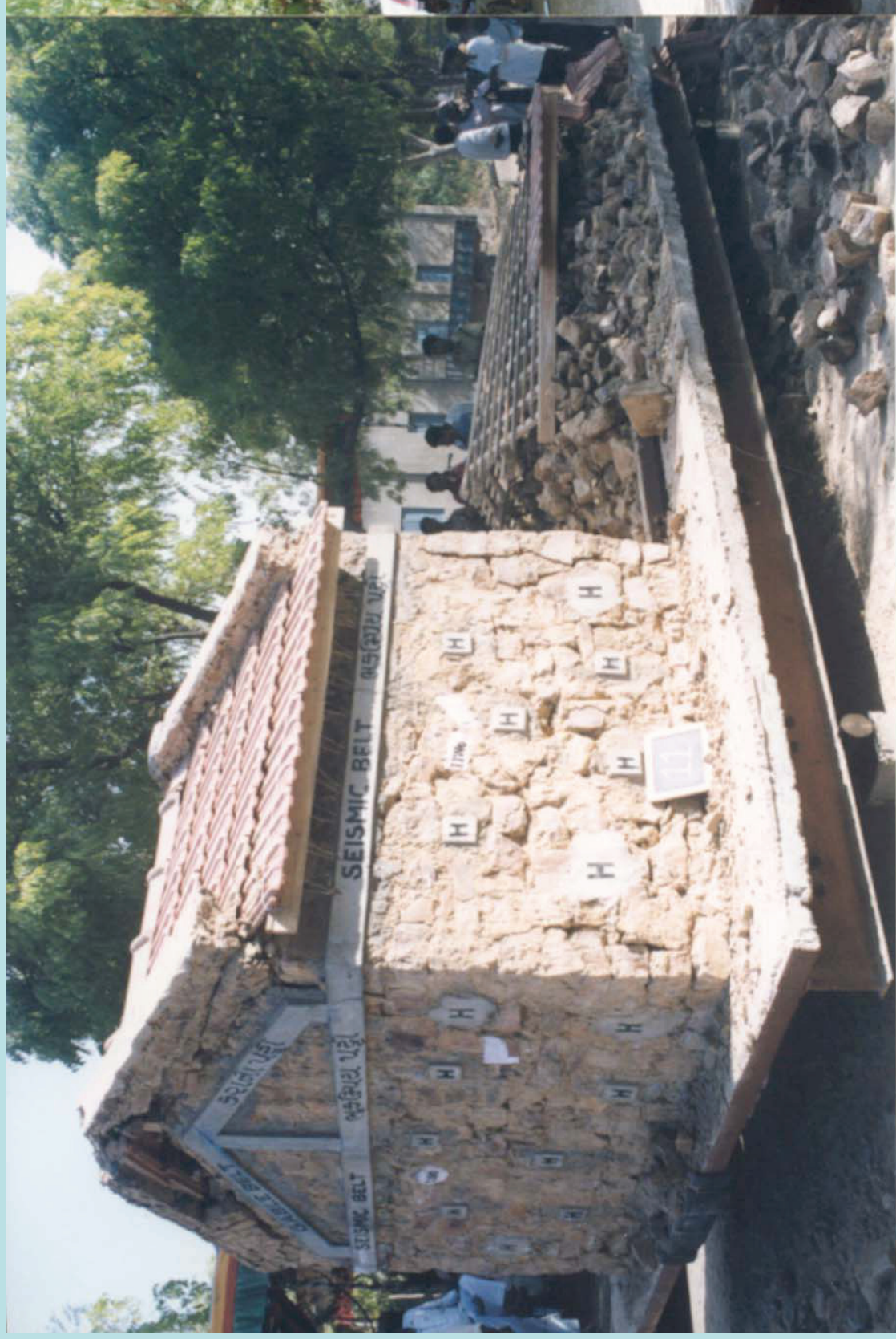
Shock No: I I ,T.M Collapse ,I.M End Wall Cracked
